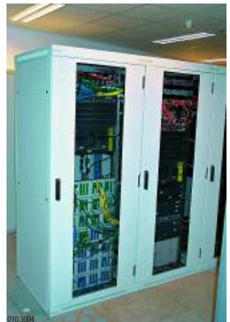
010.3004 Compact and neat: distribution cabinet with components from R&M.
