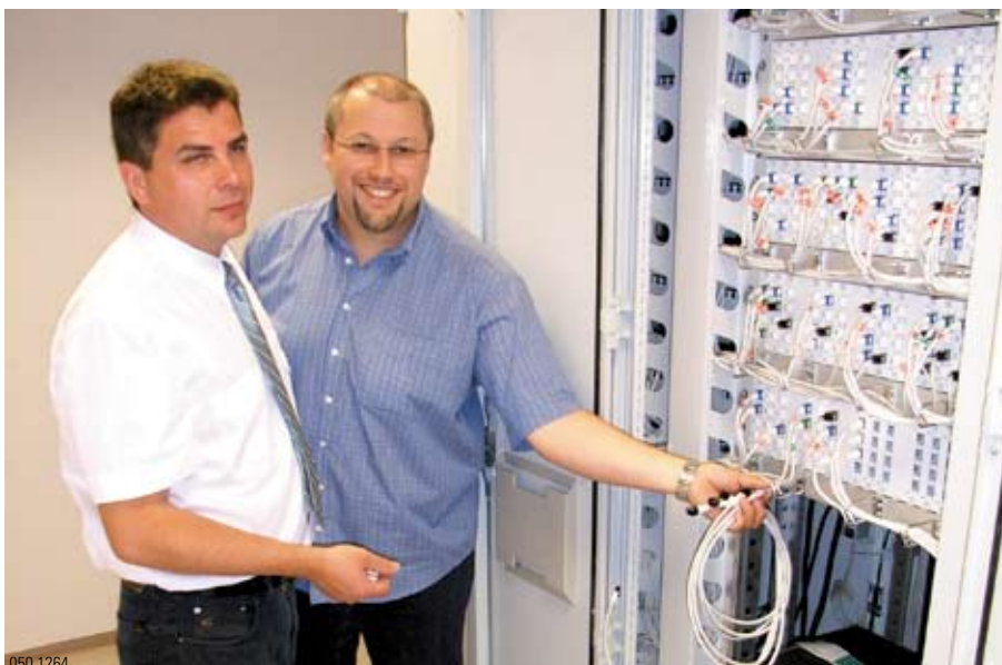
(from left to right) Mr. Müller of EDF GmbH and Mr. Hammerschmidt of Wieland-Werke AG in front of the EDP distributor in the new building, building 8, of the Ulm facility.
