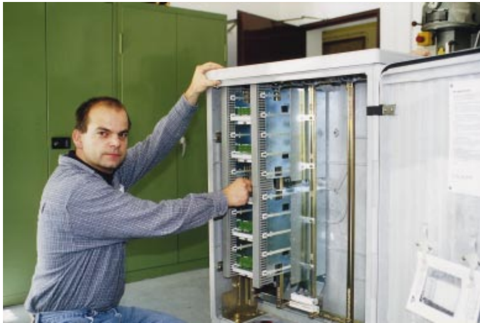
CCC housing "FiberCurb" for copper and FO
