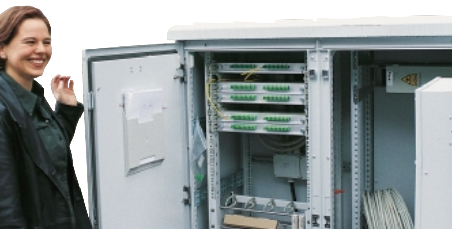
This is how the interior of an outdoor distribution cabinet looks.
